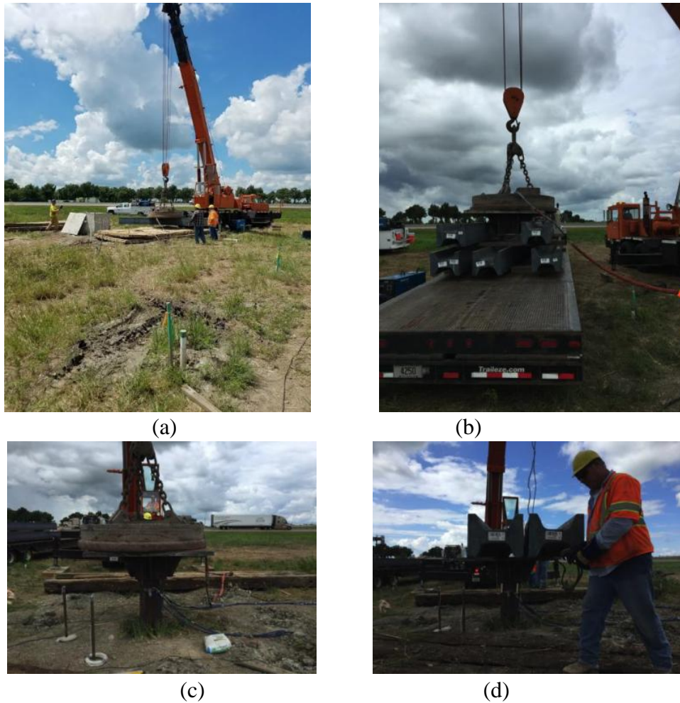
Figure A.18. Photographs of (a) the crane that was used to move the beam blanks from a truck to the H pile, (b) the steel load distribution plate being reloaded from a truck, (c) the load distribution plate being place at the top of the H-pile, and (d) the beam blanks being place at the top of the H-pile (courtesy of Richard Coffman).
