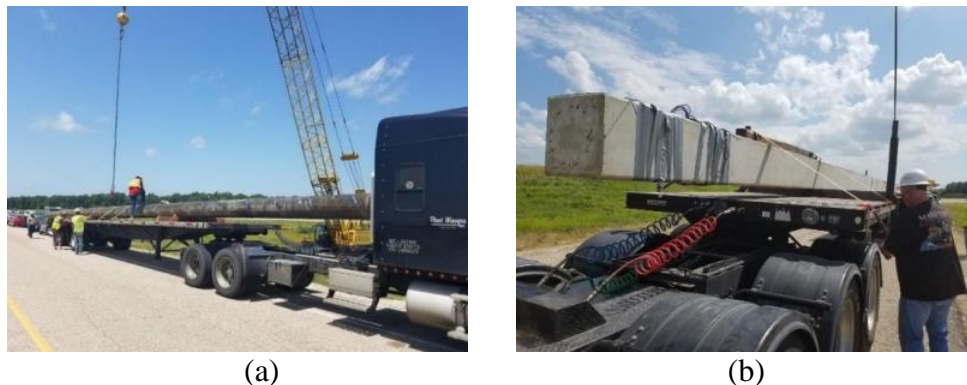
Figure A.5. Photographs of (a) the steel pipe pile , and (b) pre-stressed pile being delivered at the TATS.
